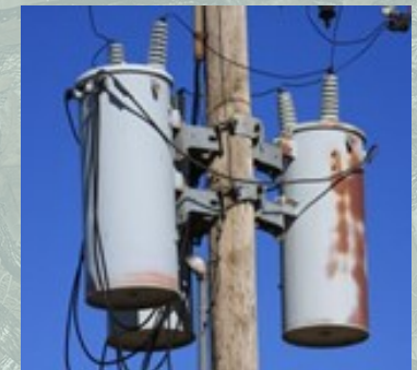
Typical PCB-containing Transformer
