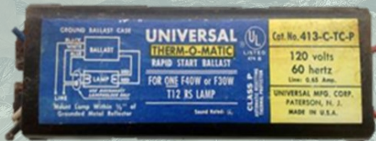
A typical pre-1979 PCB-containing fluorescent light ballast
